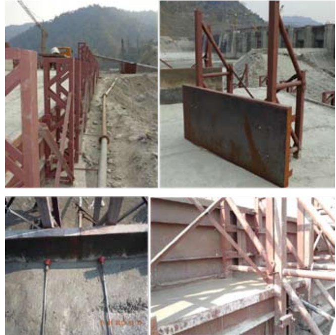
Fig. 6 : Upstream and downstream formworks (step) as used in FSTE and the anchor bolts
